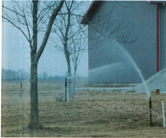
Figure 2. Onsite sprinkler irrigation system serving a three bedroom house.
